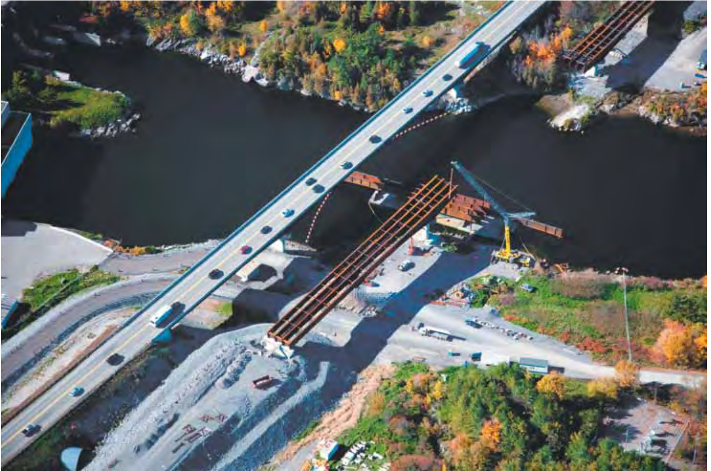
Aerial view of the centre span segments being assembled on the barge
