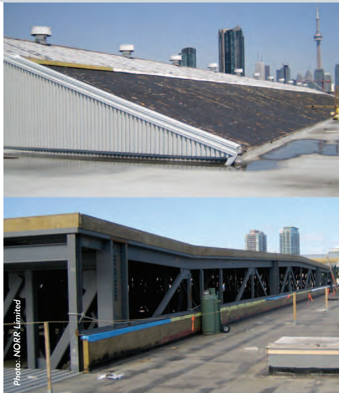
The top image shows the roof before removal. The bottom image is the result after the long-span joists were installed. The depth of the new roof integrates well with the existing structure.
