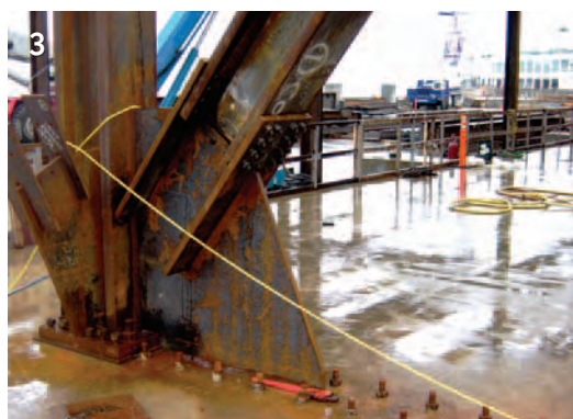
(3) Anchoring large forces into the marine deck required the bases to be cast into the deck beams. Steel templates were essential for positional control of the anchors and were used throughout the project.
