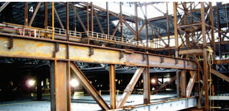
(4) Trusses span over the exhibition hall carrying the ballroom floor above and 450 car parking within the truss level
