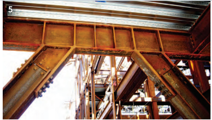
(5) Eccentric Braced Bays provide seismic and wind resistance and were placed in the few solid walls available and within service rooms causing intense coordination using Revit and Tekla software.
