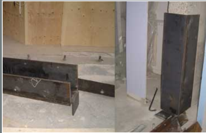
1) Bring the members necessary to build the shear plate in pieces onto the site: U-collars, W-sections, angle sections and plates.
