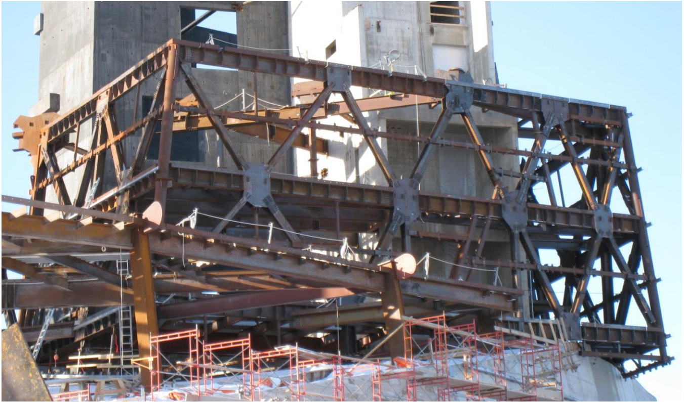
Erection of the Mountain Diagrid begins in Winter 2010 Yolles, A CH2M HILL Company
