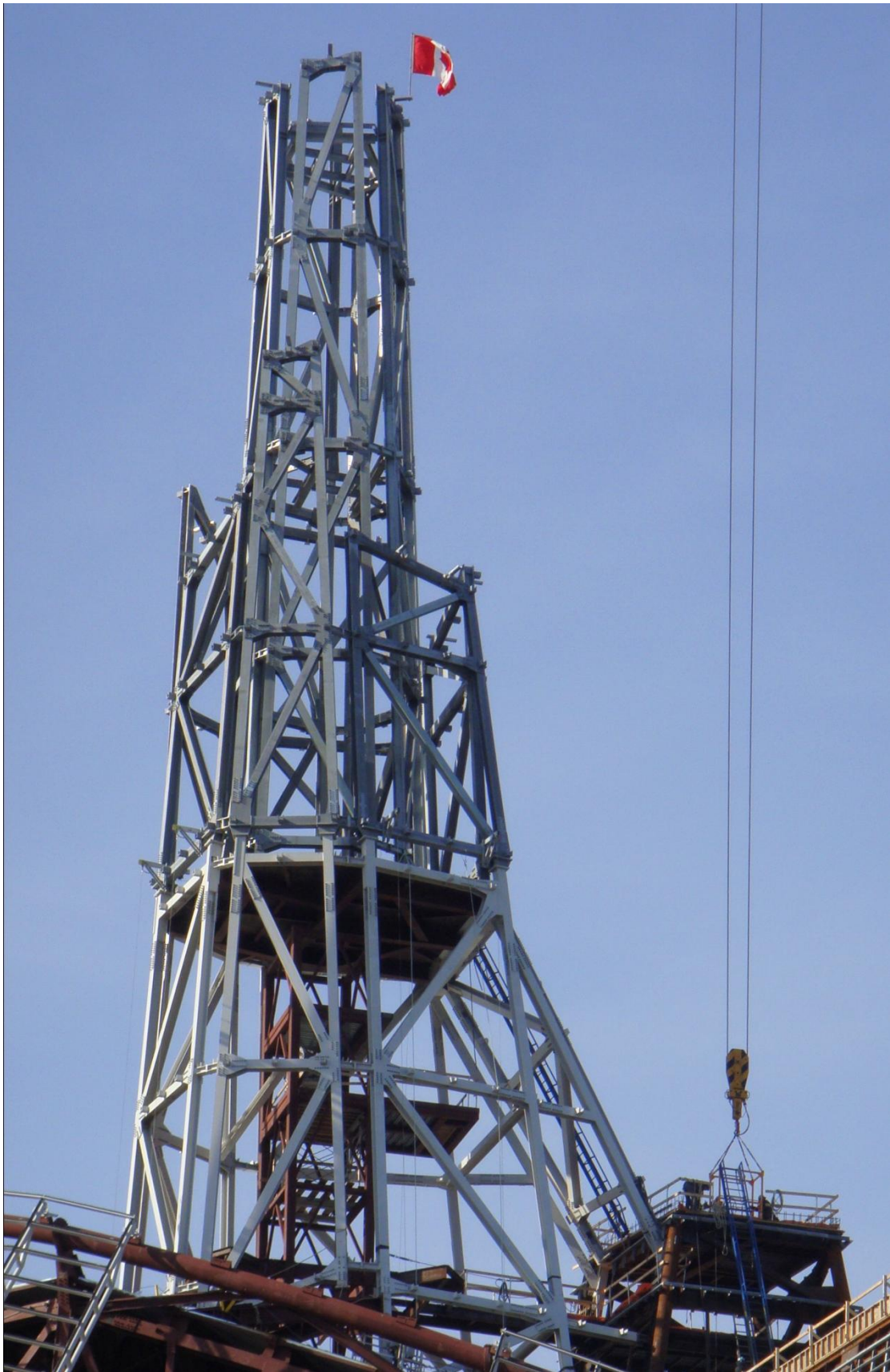
Tower of Hope Structural Steel Erection Completed Yolles, A CH2M HILL Company
