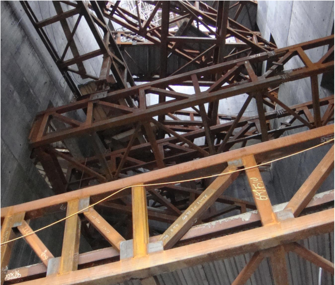
Hall of Hope Ramps in the process of installing metal deck and concrete Yolles, A CH2M HILL Company
