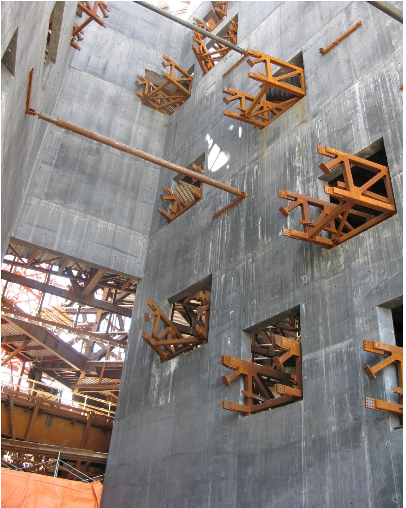
Erection of Continuous Ramps thru Hall of Hope Concrete Walls Yolles, A CH2M HILL Company
